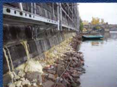
Sealing and reinforcement at the Alsovo Riverbank in Prague after the flood event in 2003
